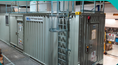
GRID POWER SUPPLY
