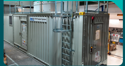
GRID POWER SUPPLY
