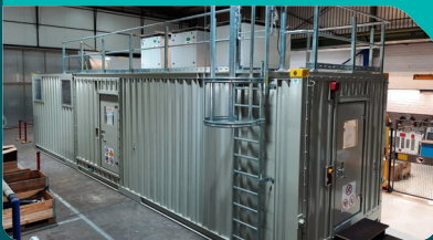
GRID POWER SUPPLY
