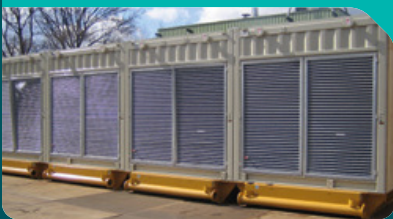
GENERATOR POWER SUPPLY
